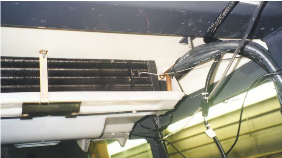
Heater tube end of evaporator coil.
